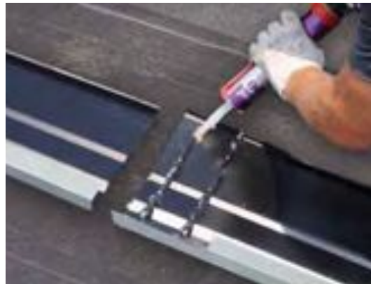
2. When overlapping, apply sealant under overlap. Be sure to screw every 12", between the diverter as shown in above diagram.
