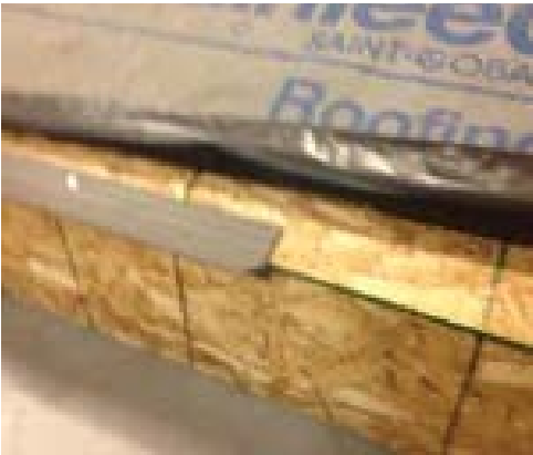
1. Cut and bend drip edge trim on the outside to conform to rake edge and inner and outer gable.
